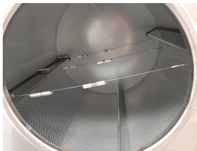
Figure 3: Installation of temperature sensors throughout dryer tumbler. 3 sensors installed in front, middle and rear sections, radially distributed to probe temperature variations from central axis to dryer wall.
